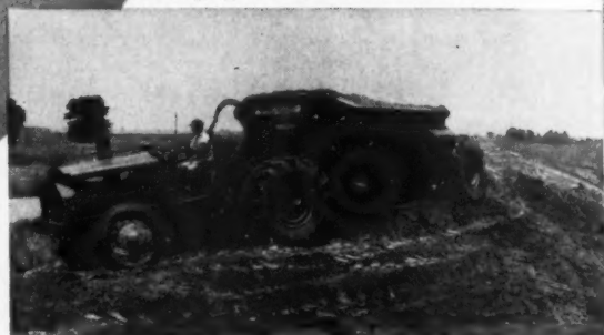
Working on a levee in Arkansas—Bottom-Dump Euclids are the outstanding choice of levee contractors.
